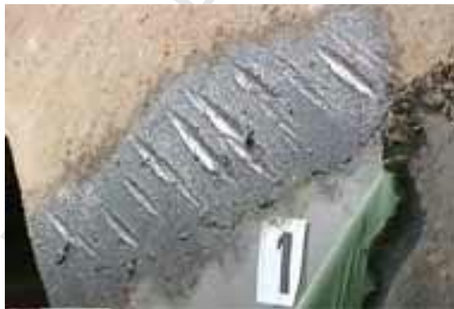
Fig 10: Example of gouges on a pipe surface provoked by a scrapers.
