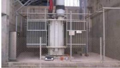
Fig.2. The studied electrical power transformer.
